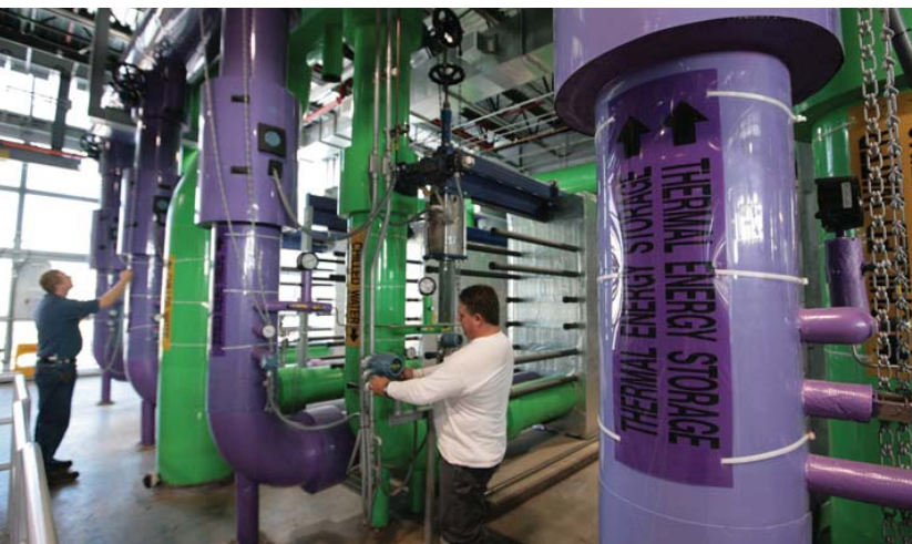
Chilled water plant
